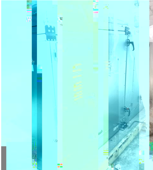
HVAC unit placed @ mechanical room
